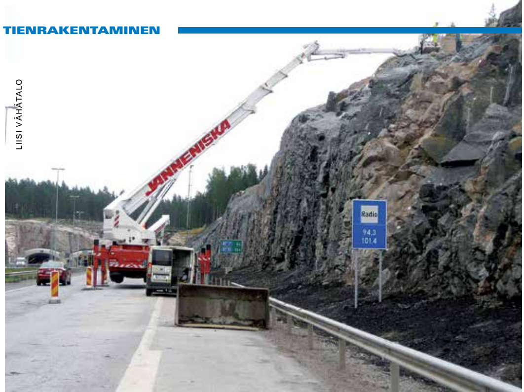
Figure 5: Cleaning up the damages caused by the fallen down boulders on the motorway E-18. Boulders were fractured off from the rock cliff due to thermal stresses.
