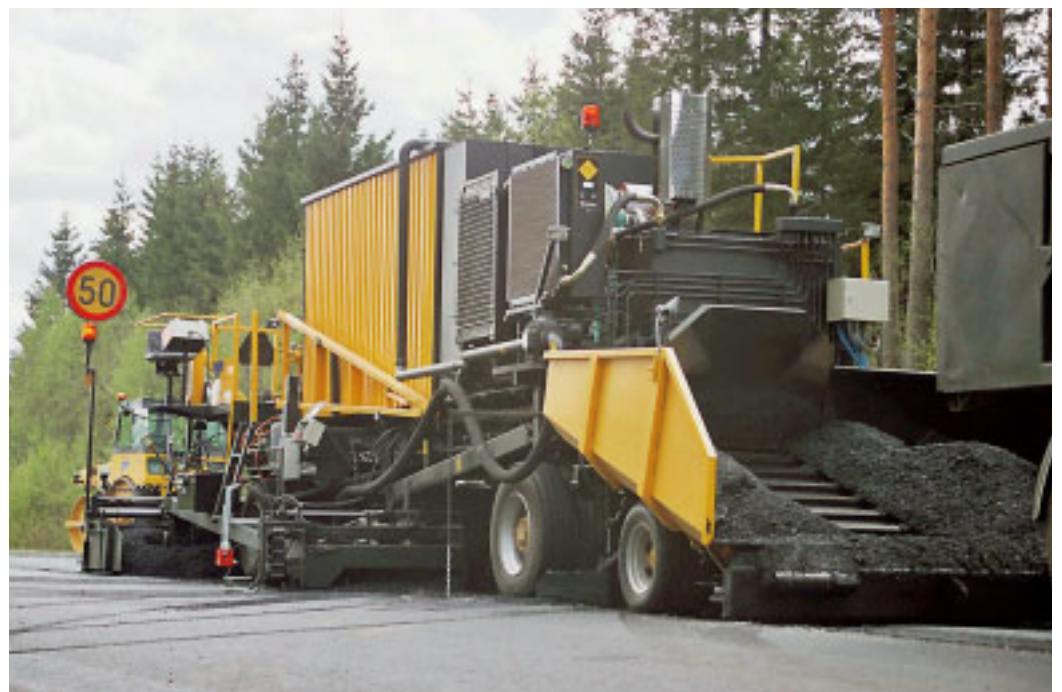
Funding for pavement repair and patching has been increased in recent years, but the need is expected to continue growing strongly.
